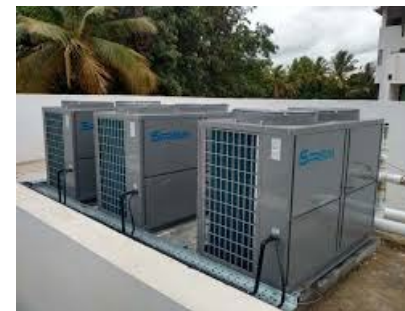
Roof mounted air source heat pumps
