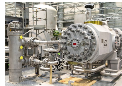
Example: large scale heat pump in an energy centre
