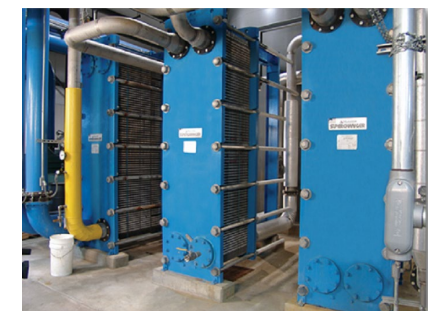
Heat Exchanger serving a large building
