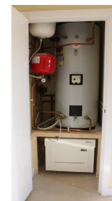
Individual heat pump and hot water tank in each dwelling
