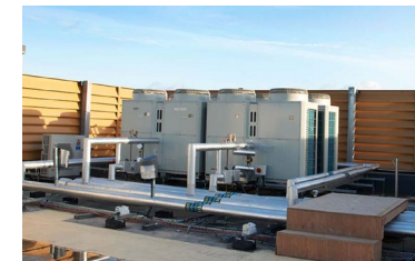
Communal rooftop air source heat pumps
