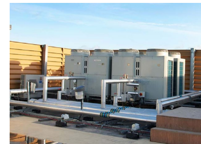
Example: communal rooftop air source heat pumps
