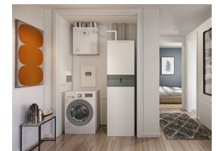
Individual heat pump in each dwelling
