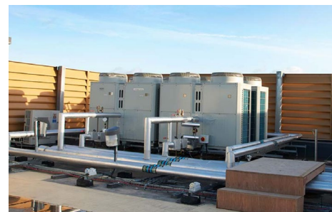
Communal rooftop air source heat pumps
