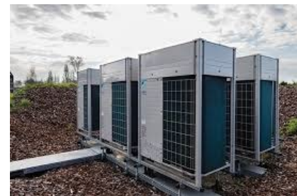
External condenser units
